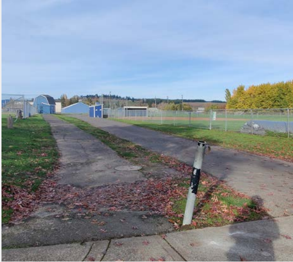
On the west side of the District-owned access road, a paved shared-use path connects the Elementary School to the Middle and High School.
