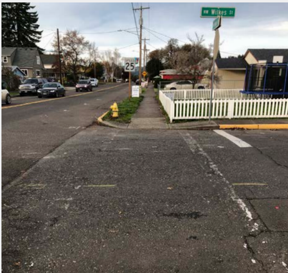
At Wilkes St and Highway 47, the crosswalk has faded.
